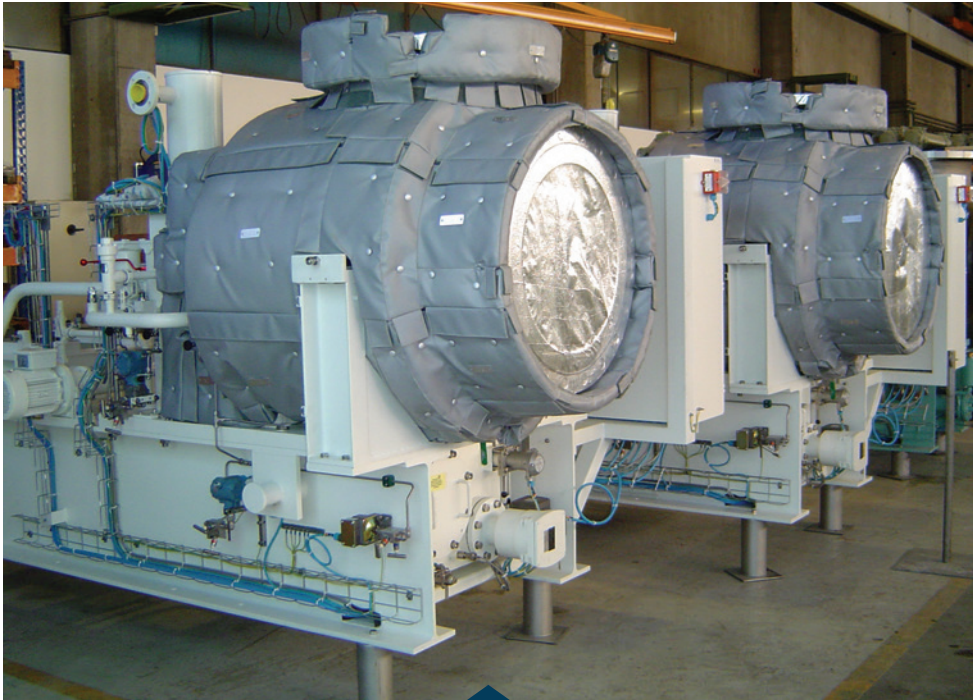
Single stage return gas blower
